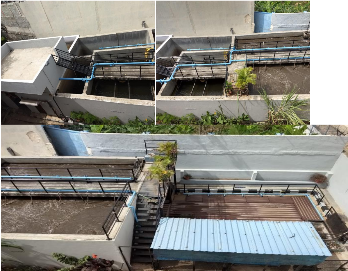
(2) 7 KLD e-SBR Technologies STP.
